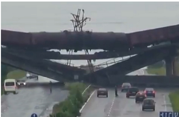
The destruction of a railway bridge in Donbass, 25 July 2014. Source: Wikipedia
